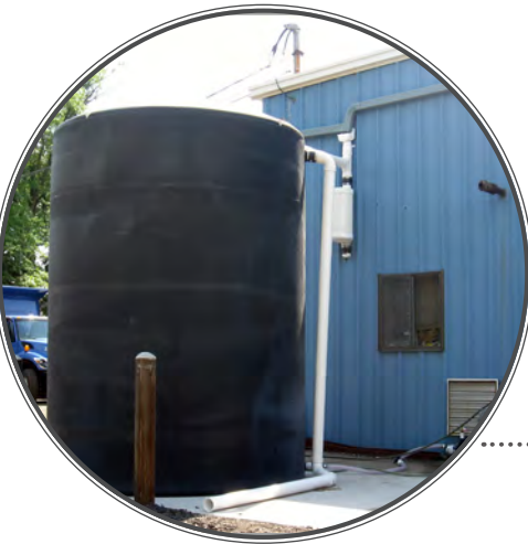
LOCATION: Clark, NJ This cistern was installed at a public works department. The rainwater is harvested from the rooftop of the building and used as part of a “green car wash” system that uses rainwater.
